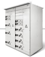
Low Voltage Switchgear & Motor Control Center
